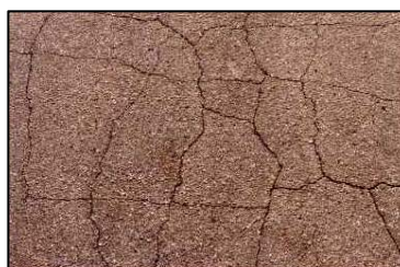
Condition 5 – Very poor
