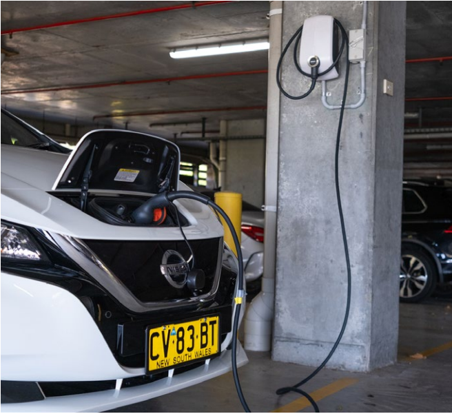
Our electric passenger vehicles charging at Town Hall House. Credit: Chris Southwood
