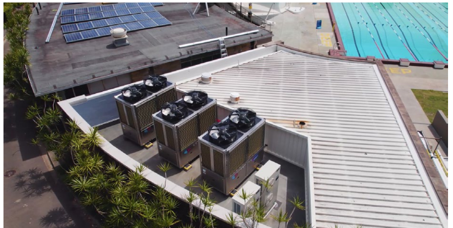
Electric heat pumps replacing gas at Victoria Park Pool. Credit: Supplied by Image Air
