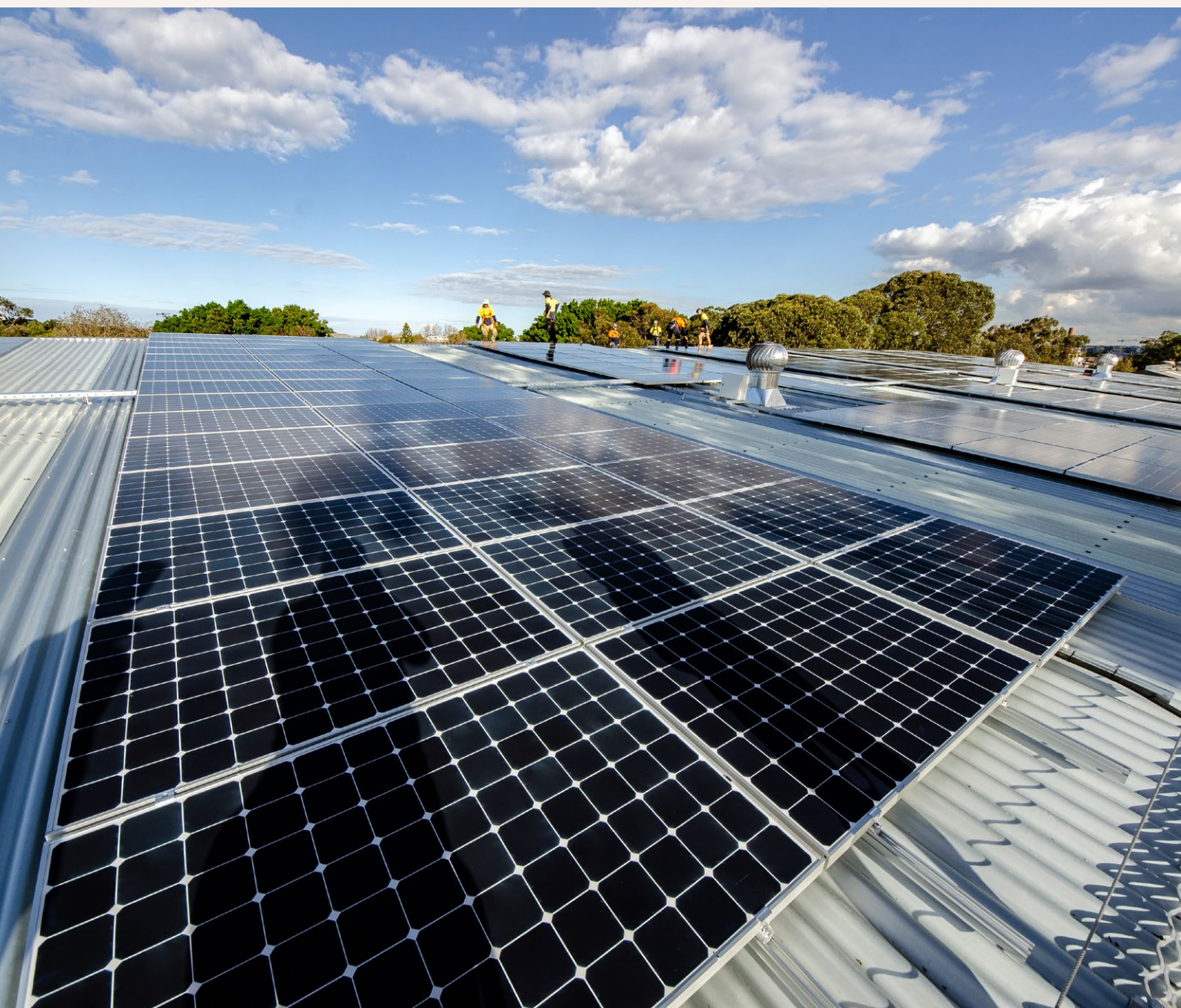
Rooftop solar panel array at Perry Park Recreational Centre, Alexandria. Credit: City of Sydney
