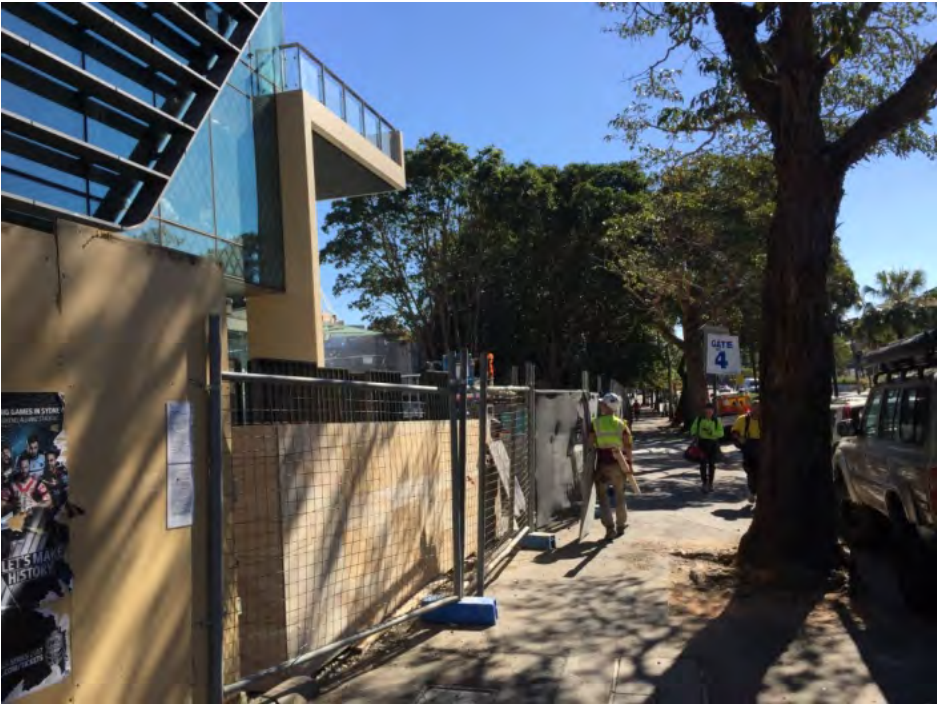
Plate 3.4 Location above the alignment of Busby's Bore showing current construction zone (view west)
