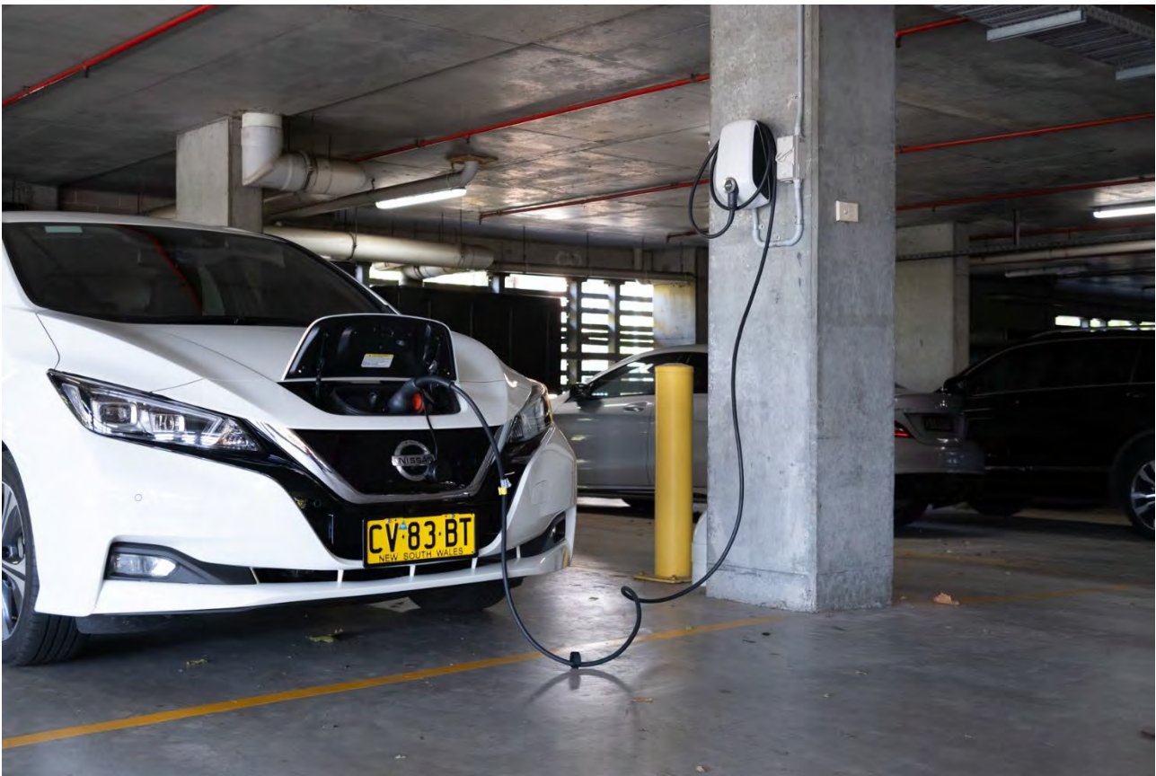
Charging point at the Goulburn Street parking station (Photo by Chris Southwood / City of Sydney)
